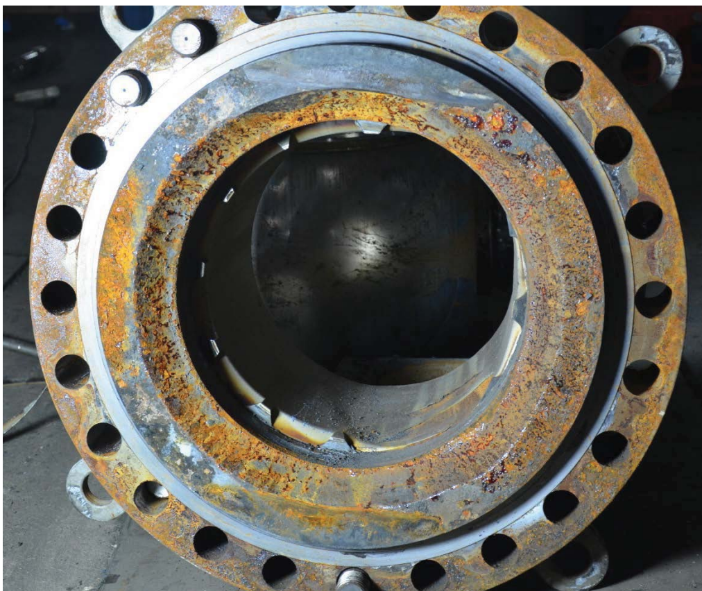
阀门通道严重冲蚀
